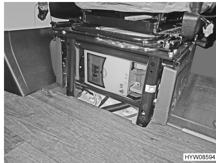
Fig. 53 Location of 240 V fuse box
